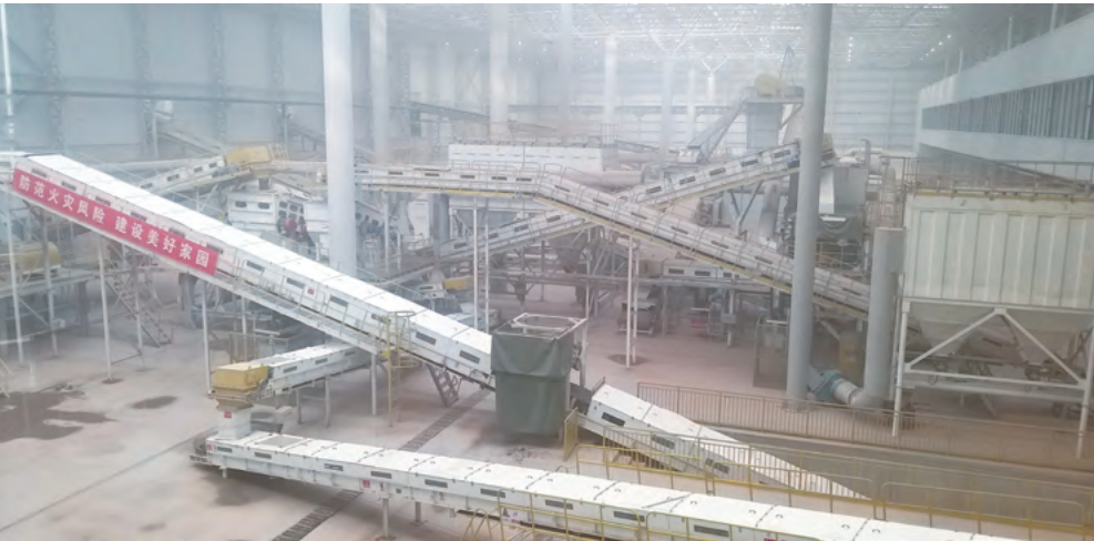
Closed-circuit management, preventing leaks and fugitive emissions
