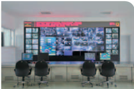
Central Control Room of Aoniu Mine 1st Processing Workshop
