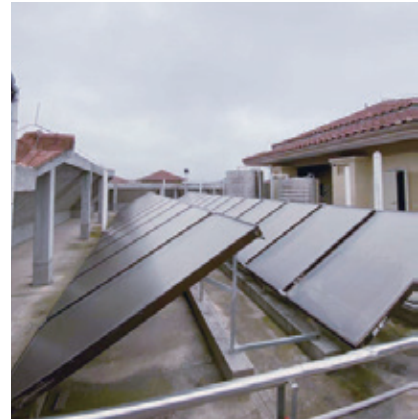
Solar water heating system
