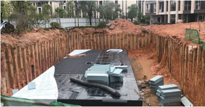
Rainwater recovery system
