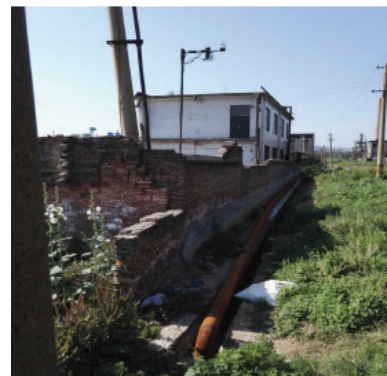
Figure of video monitoring of the main drainage outlet of No. 1 sub-plant
