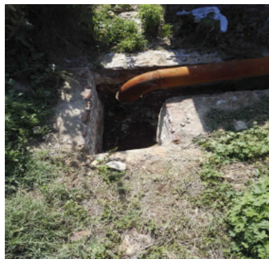
Figure of blocking the main drainage outlet of No. 1 sub-plant
