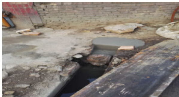
Figure of blocking the east drainage outlet for domestic water of No. 3 sub-plant
