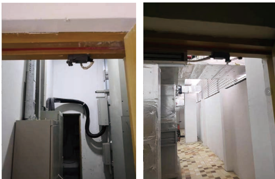
(Install on-line switches for all equipment rooms, light on the door, and turn off the door)
