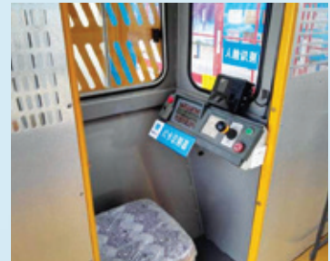
Driver of construction elevator face recognition system
