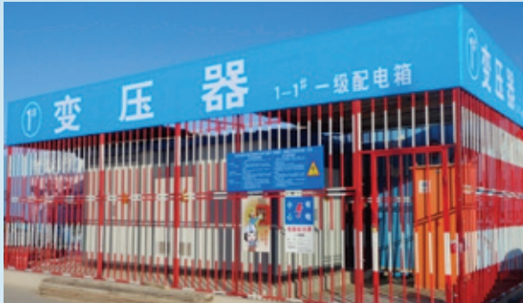
Protection for box transformer
