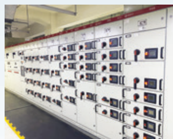
The power distribution room of AsialInfo Plaza after transformation
