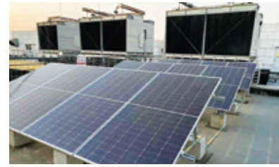
Photovoltaic facilities on the top floor of AsialInfo Technologies Plaza
