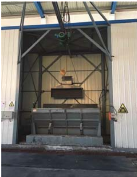
Feed Inlet of Pre-treatment
