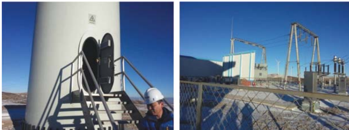
Figure 7.3 Examples of Site Plant Equipment (Typical Wind Tower Structure and Power Switchgear System)
