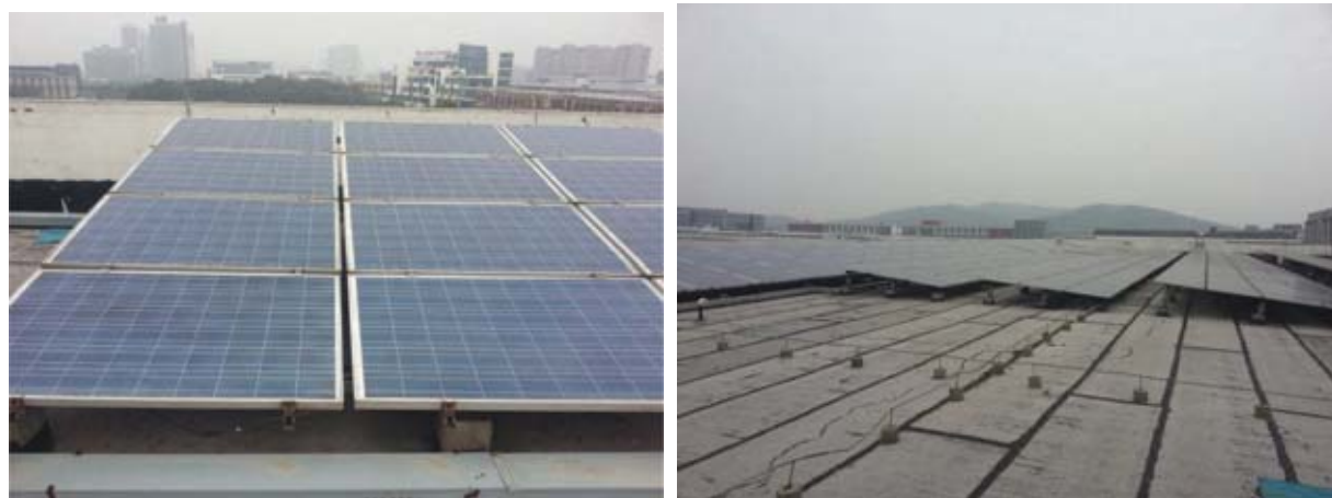
Figure 6.4 Photovoltaic (PV) Module Arrays
