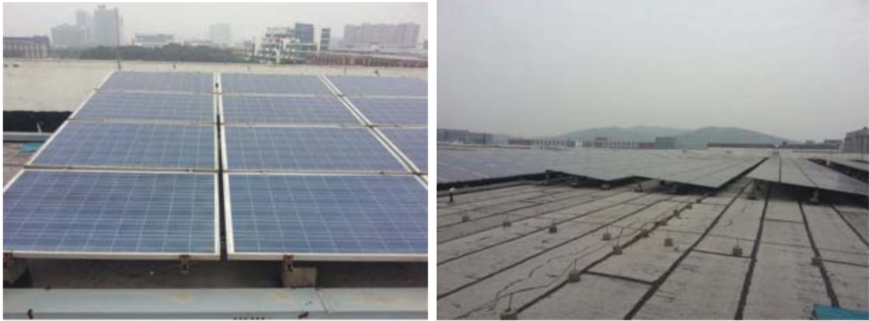
Figure 6.4 Photovoltaic (PV) Module Arrays
