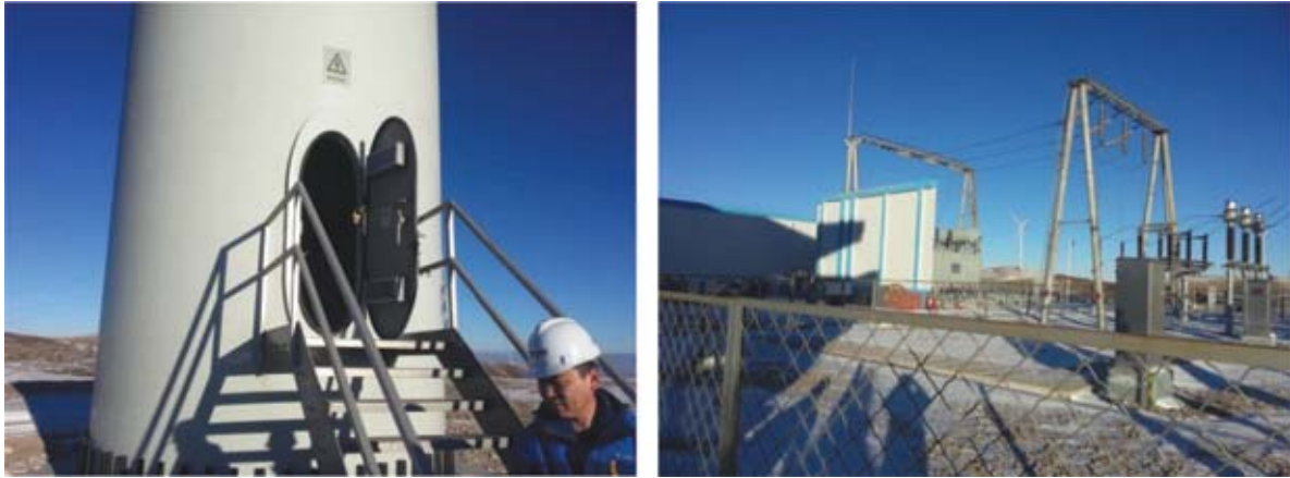
Figure 7.3 Examples of Site Plant Equipment (Typical Wind Tower Structure and Power Switchgear System)
