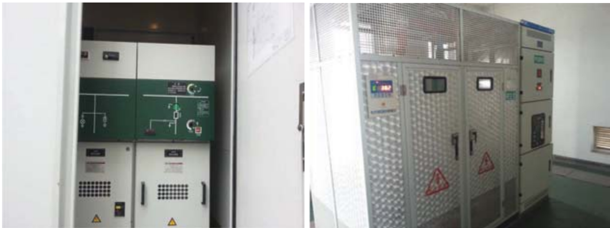
Figure 6.3 Examples of Site Plant Equipment (Typical Inverter and Electrical System)
