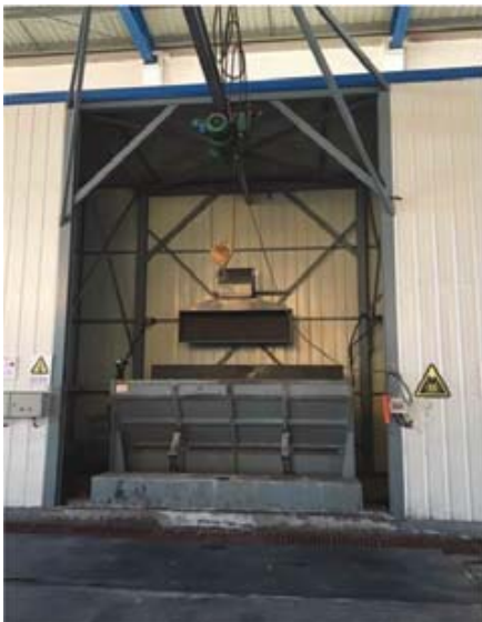
Feed Inlet of Pre-treatment
