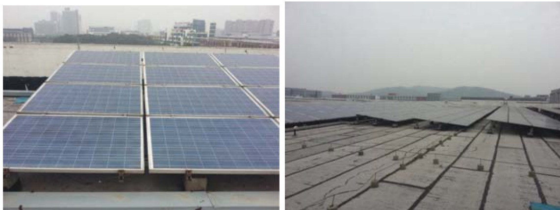
Figure 6.4 Photovoltaic (PV) Module Arrays
