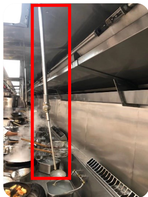
Figure 3b – The sensor installed on the furnace
