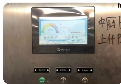
Figure 3c – Transformer and system monitor
