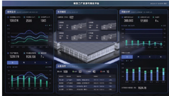
Smart energy system — monitoring console of the whole plant area
