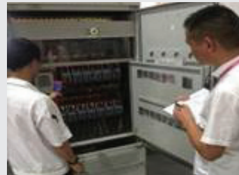
Special inspections of power distribution cabinets
