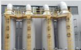
Wet dust removal
